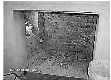
Badly Deteriorated Firebox
