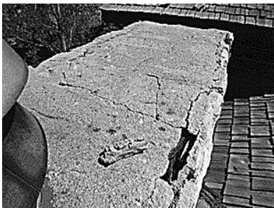
Damaged Chimney Cap
